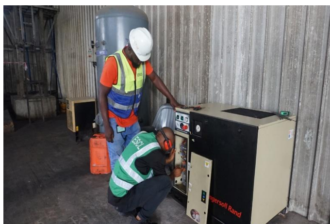
Maintenance (Compressor) Unit
